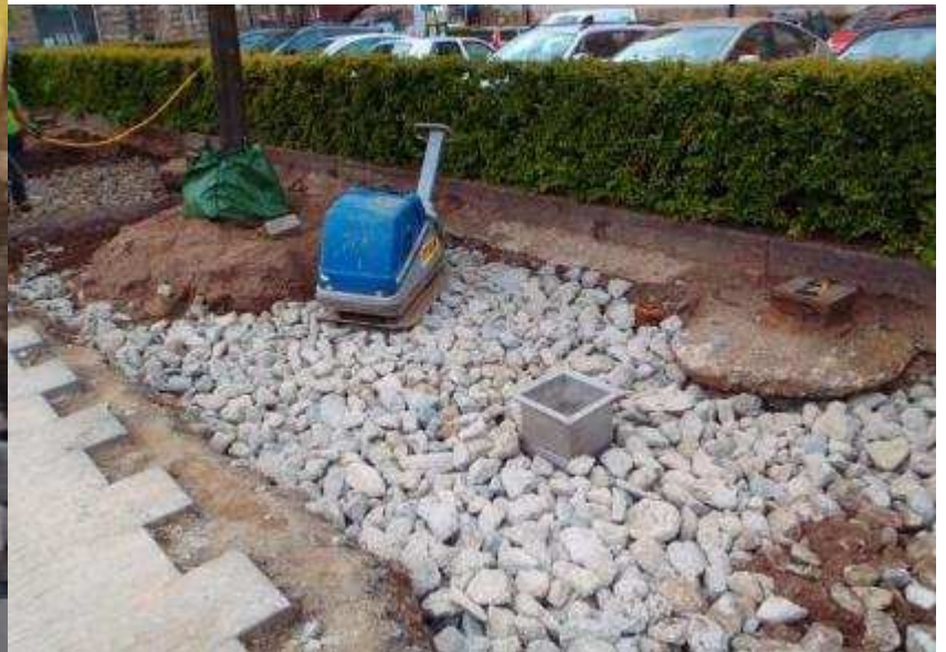
Recycled concrete used as a part of the structural soil instead of granite
