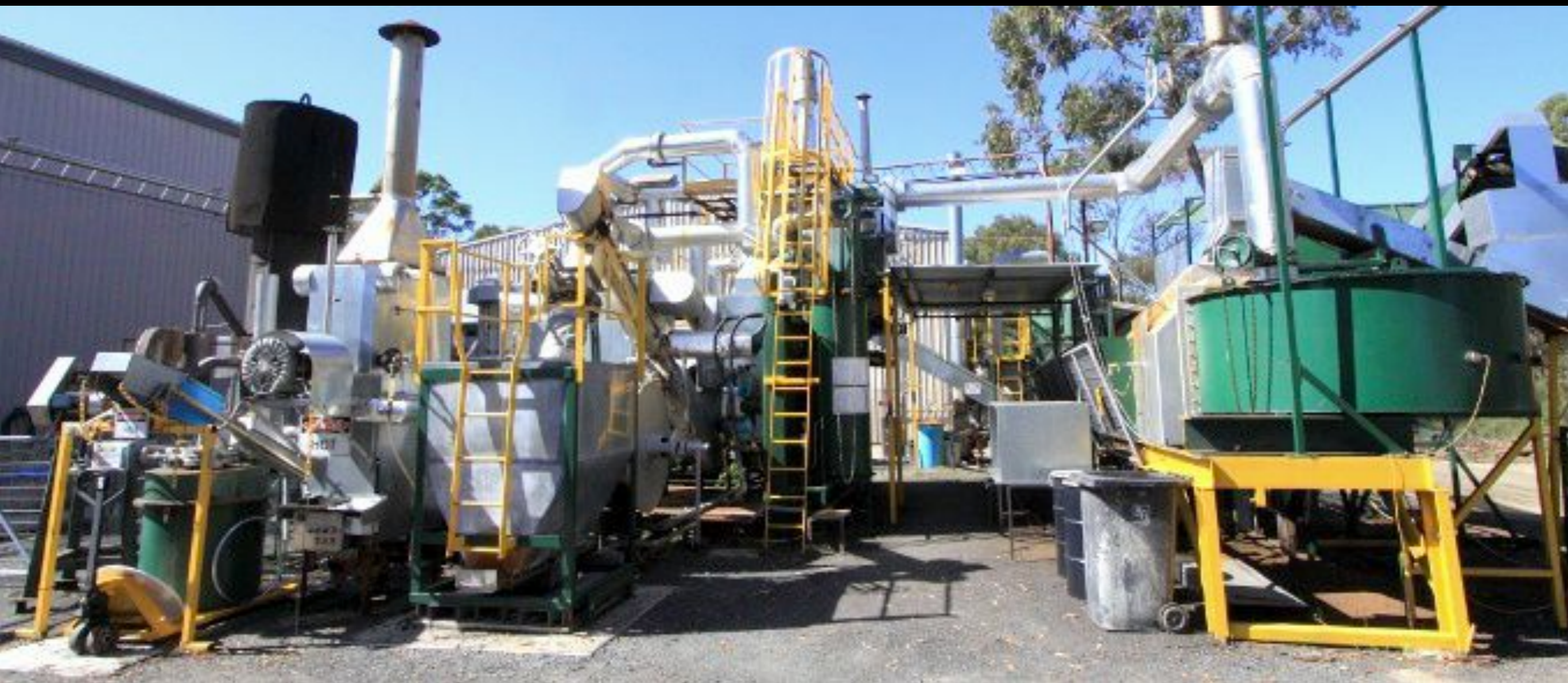
Pacific Pyrolysis pilot plant Capacity 300 kg/hr biomass
